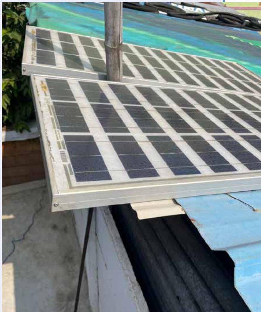
.IMAGE 2 | Solar PV Panels at Installed at Jagan's Workshop
